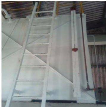
Figure 1. Mechanical tank liquid level indicate systems
